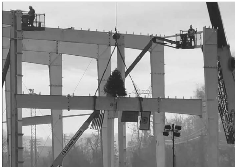
Workers at the Form Energy project in Weirton, West Virginia raise the final structural beam, marking a major milestone in the construction of the project.
