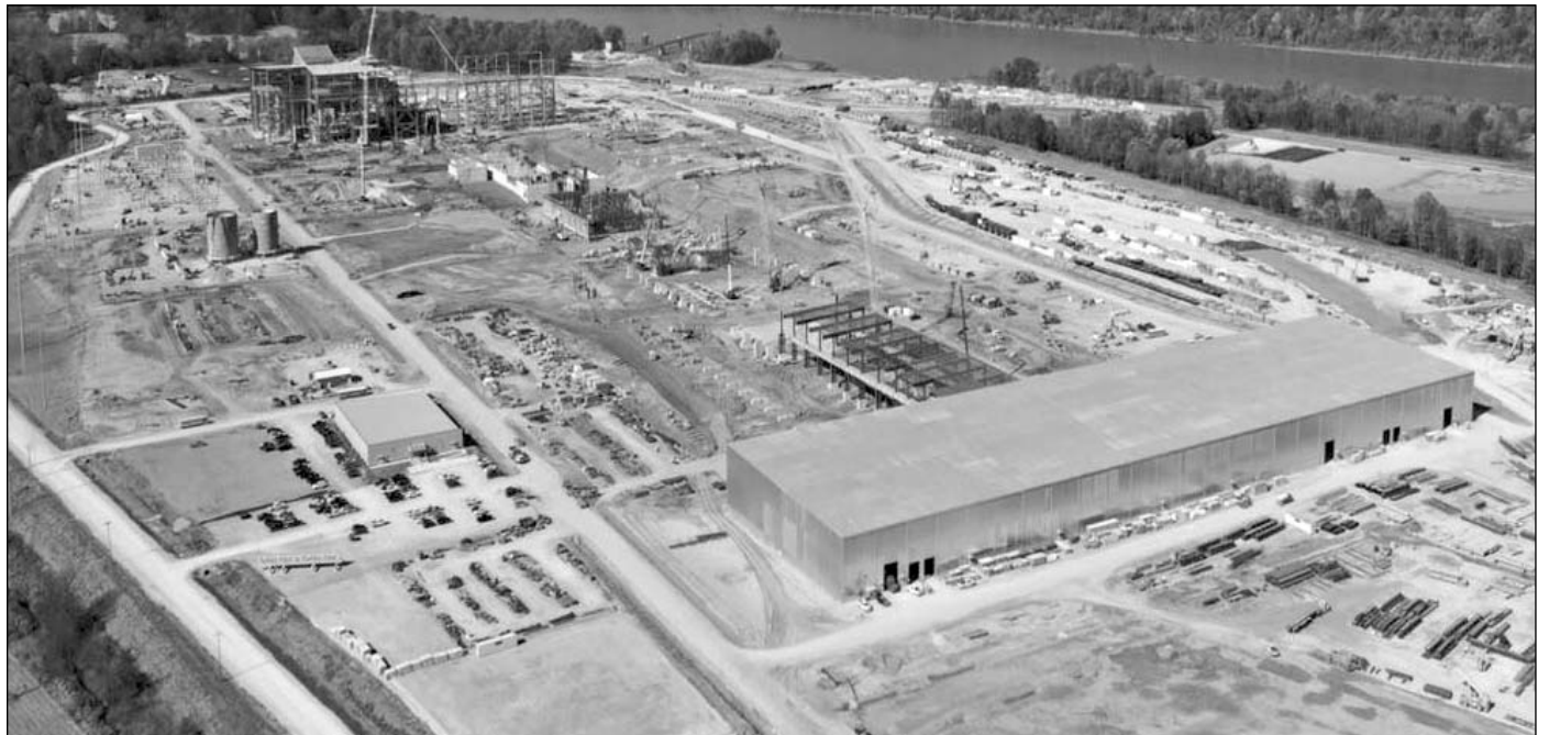
This Nucore facility in Brandenburg, Kentucky is still under construction. Reports suggest out-of-state workers make up over 80% of the total project workforce. With the recent award of a concrete contract to out-of-state contractor ABC Concrete at the Mason County facility, who is also working on the Brandenburg project, it is likely the West Virginia project will have the same result.
