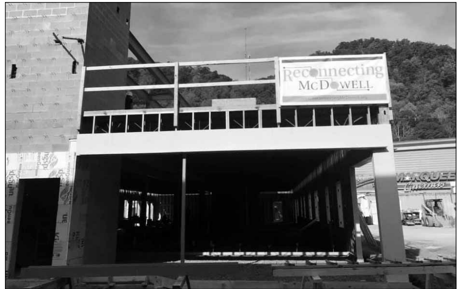
A formal groundbreaking event was held in Welch on September 9 for the $8 million Renaissance Village housing project. The project, which is already well underway, will provide rental housing for public school teachers. BBL-Carlton is the GC on the all union-built job.
