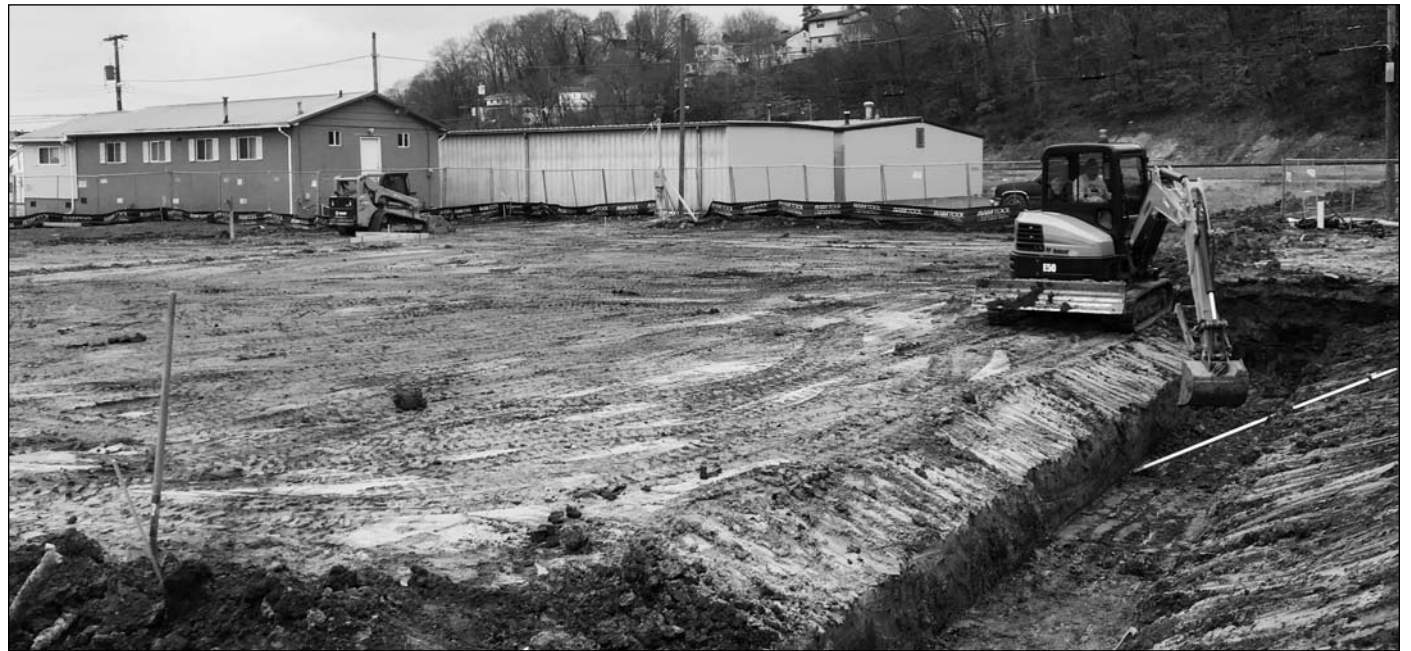
The Apprenticeship program for IBEW Local 466 in Charleston has a new hands-on training facility under construction. The 50' x 60' building will have 20 foot ceilings and an open floor plan for flexible training mock-ups. The project is expected to be complete later this year. MIRC Construction Services of Charleston is the general contractor.
