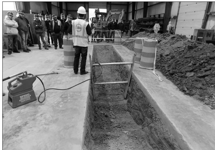
Laborers Training Instructor Corey Dornon shows members how to properly inspect a trench according to the OSHA standard and install various types of trench protection. The session was part of a new two day Pipeline Construction Safety Class aimed at protecting worker health and safety and was held at the Laborers Training facility in Mineral Wells.
