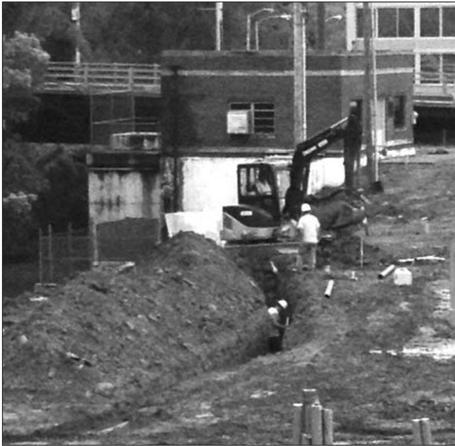
Terry Turley, Business Representative for Electricians Local 466, noticed this worker in a trench with no shoring or protection and knew right away it was a dangerous situation. OSHA fined Hi-Tech Electric $9,000 for numerous violations including the lack of shoring at the site.
