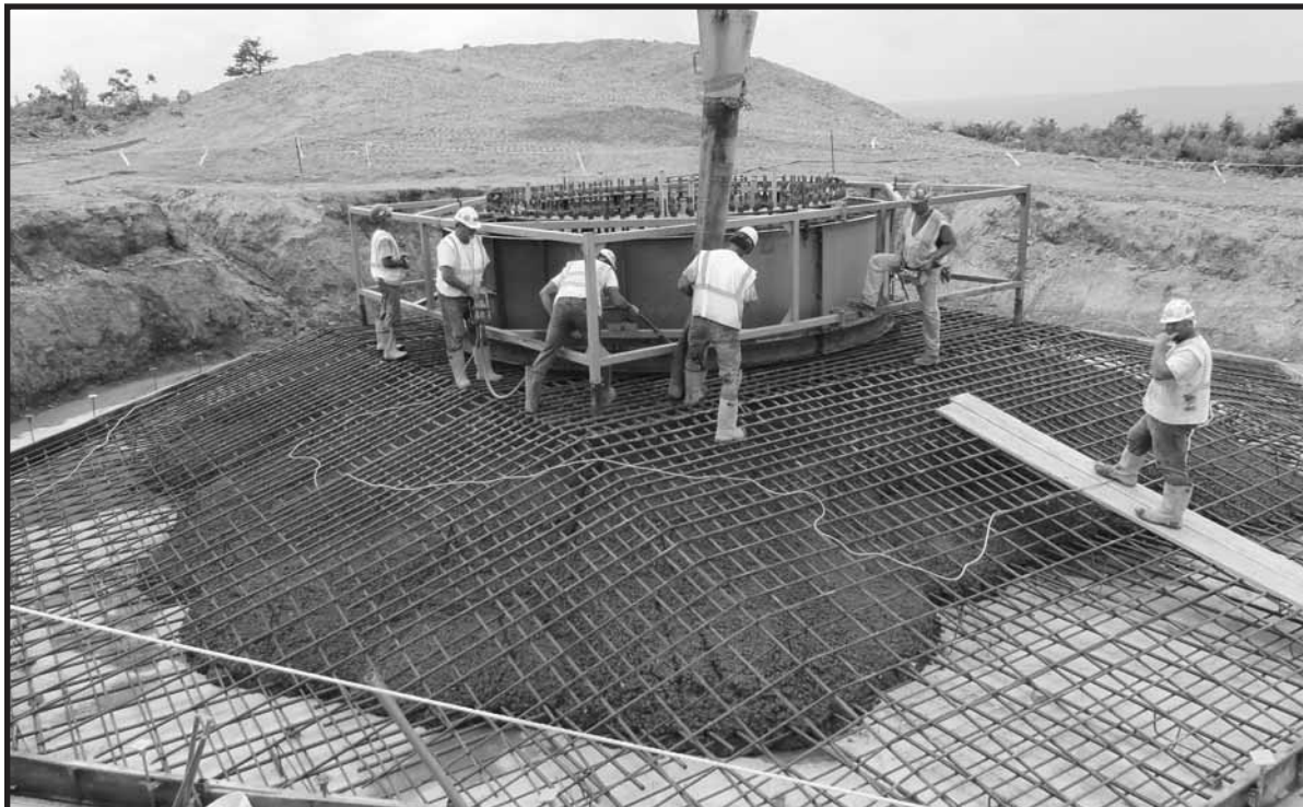
WORKERS PLACE CONCRETE at for the base of a turbine at the 23 wind turbine Pinnacle Wind Farm project in Mineral County. Each tower base required 350 cubic yards of concrete.
