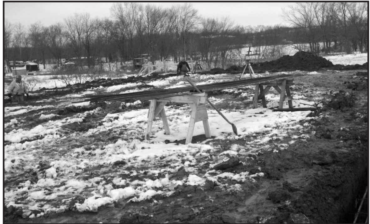
BUILDING A NEW training center in Parkersburg for Plasterers & Cement Masons Local 926 are union workers from Agsten Construction.
