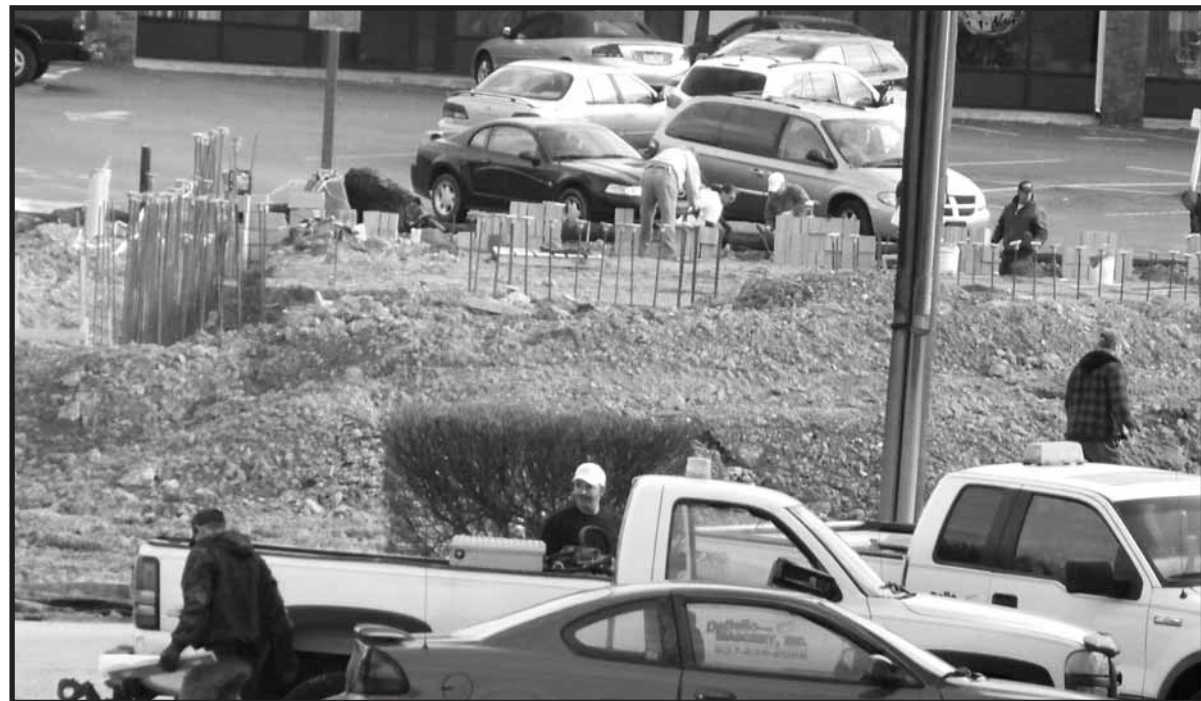
DEBELLO MASONRY STARTED work on this AutoZone in Cross Lanes. After they defaulted on payments to the Insurance Commission and were shut down the company started a new corporation, D & N Masonry, and kept on working.
