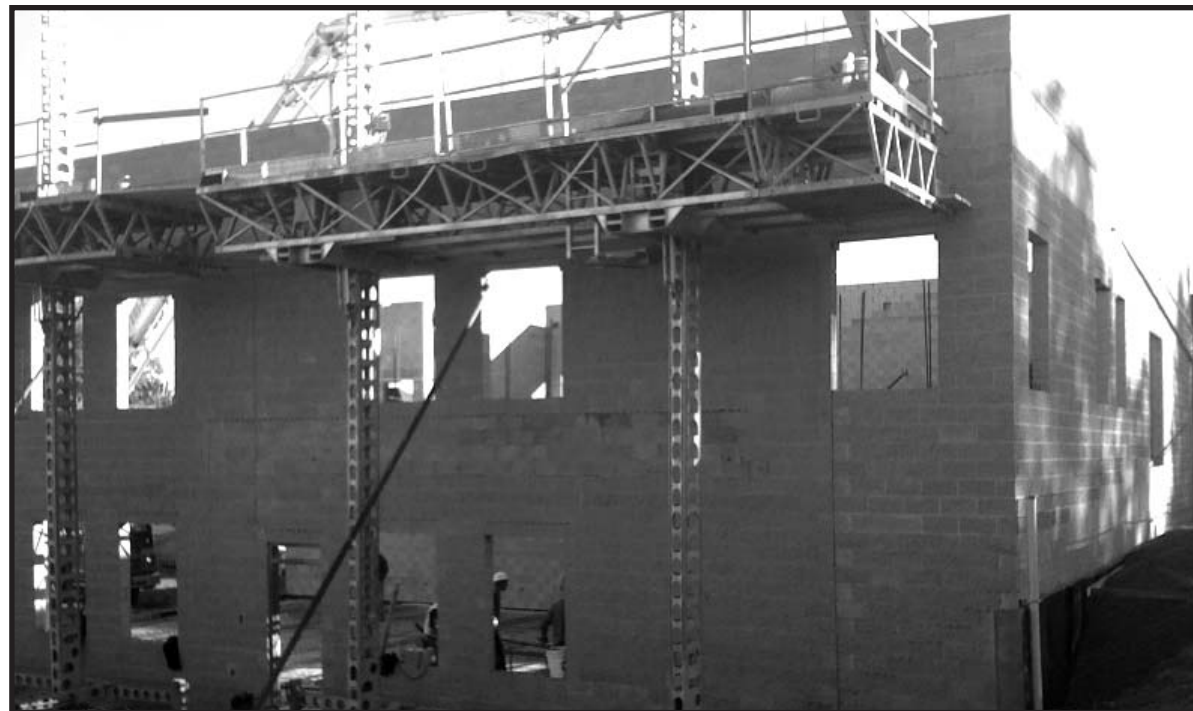
PICTURED LAST FALL is the new Apprenticeship building under construction for IBEW 317. The $1.2 million building was completed in May.
