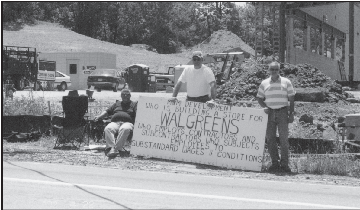
LETTING THE PUBLIC know about sub-standard conditions at Walgreens are Bill Taraczkozy (left) and Henry Neal (right) of the WV Laborers District Council and Robbie Church of Operating Engineers Local 132 (center).
