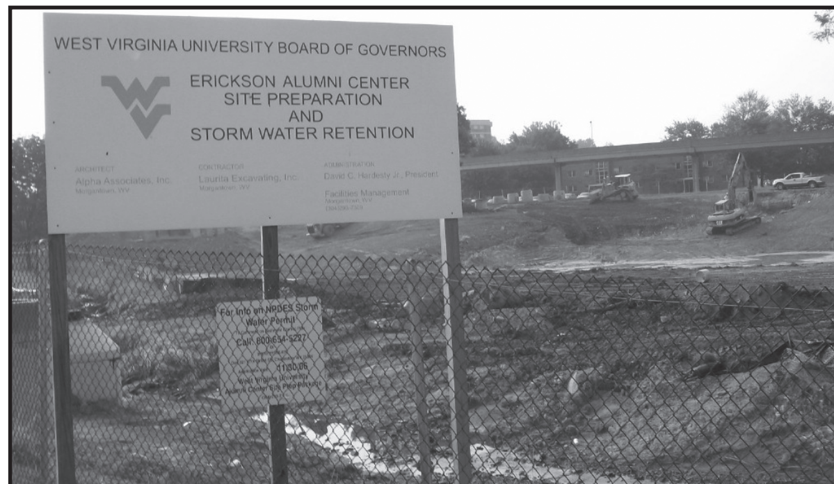
WVU PAID FOR this site preparation and foundation work for the Alumni Center but now says the project is private and not subject to bidding or wage laws.
