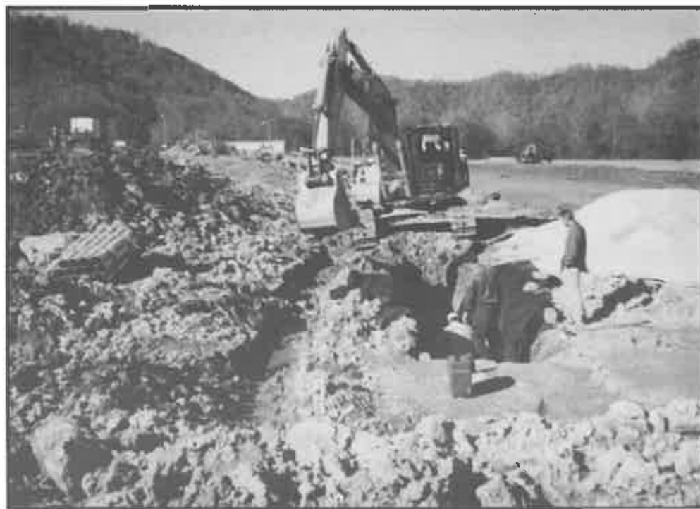
Radford & Radford workers connect pipe in dangerous, unsecured 10-foot trench at the Wyoming East High School site.
