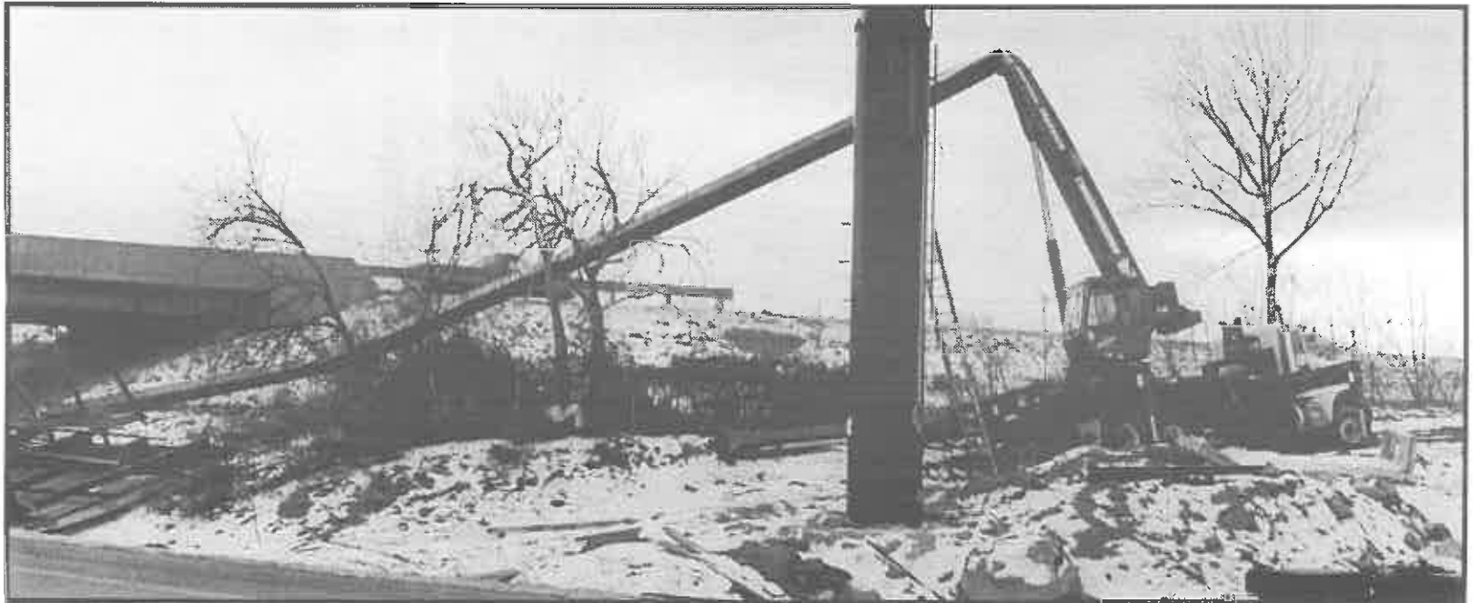
It is unclear what caused the crane's boom to buckle and drop this billboard near I-81. Another 10 feet could have meant disaster had the sign fallen on passing traffic.
