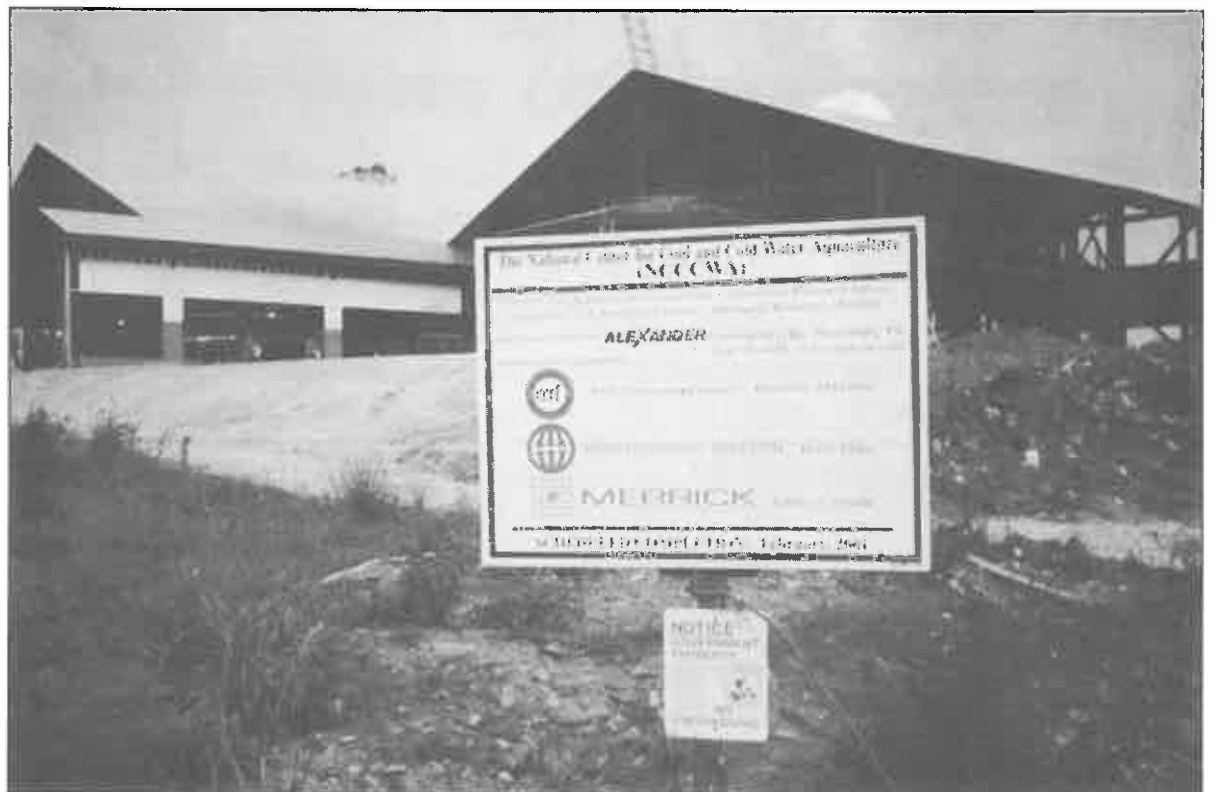
The National Center for Cool and Cold Water Aquaculture near Martinsburg now is being constructed by union workers. Pictured above is the work site where Alexander Constructors is the major contractor.
