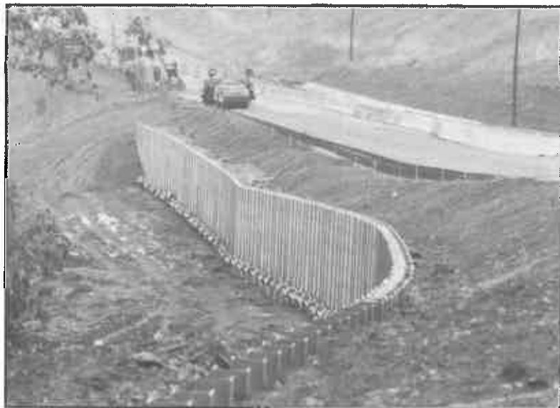
NOT SLIP-SLIDING AWAY . . . A landslide on Rt. 33 near Cottageville in Jackson County was fixed by union workers. The job required pre-drilling set beams 10 feet into rock and installing 53 tieback anchors 135 feet long. It was paid for with $1.35 million in federal funds and $338,531 in state funds. Gary Tillis, ACT's fair contracting representative, monitored it.
